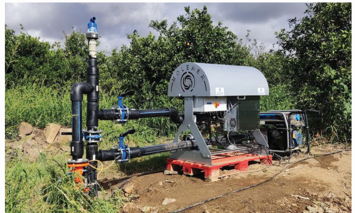
Moleaer INDALO G installed on the irrigation headworks at Cítricos del Andévalo, June 2024.
