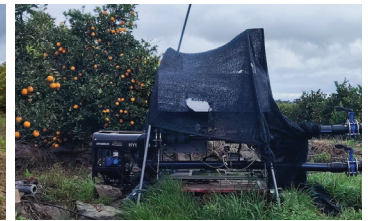
Treated parcel, January 2025. Heavy fruit load on adjacent trees, with the INDALO G unit at the irrigation header.
